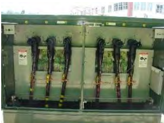
Line Side of Deadfront Switchgear
