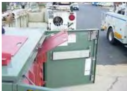
Fuse compartment barrier fully inserted
