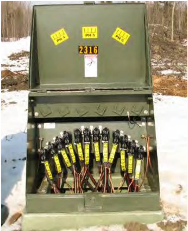
PADMOUNTED JUNCTION ENCLOSURE
