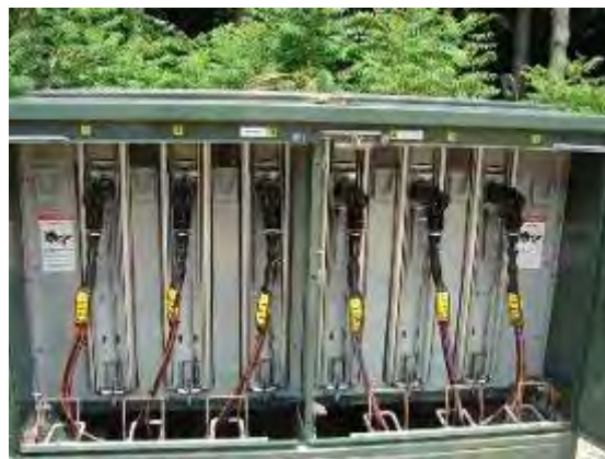
Load Side of Deadfront Switchgear
