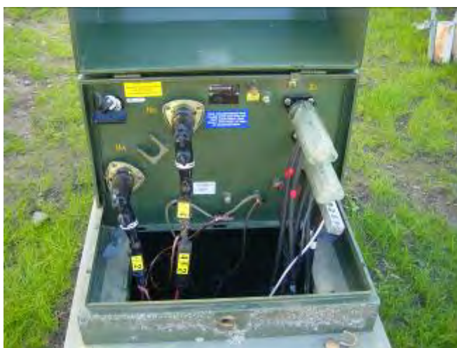
SINGLE PHASE PADMOUNTED TRANSFORMER
