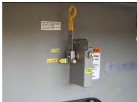
Vacuum Load Break Switch
