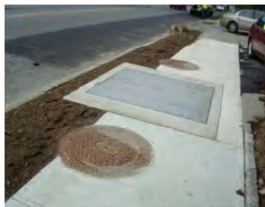
Standard item UM31 installed in side walk
