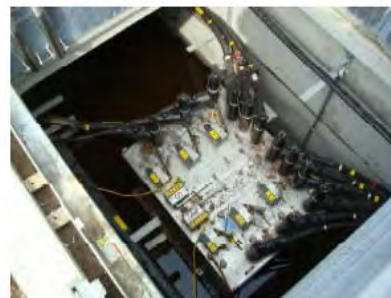
Switch installed in manhole
