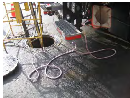
Cable Truck Grounded to Ground Grid
