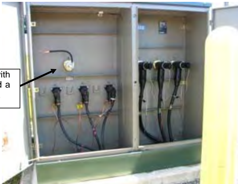
Figure #4 – Dead-front pad-mounted transformer with live-front H0 bushing
