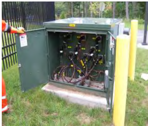
PRIMARY METERING CABINET
