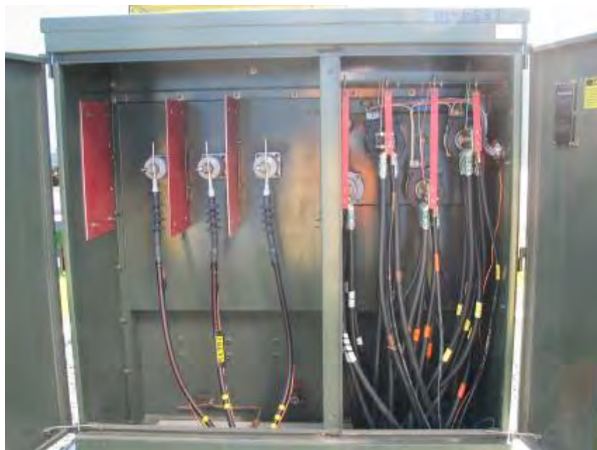
LIVE FRONT 3 PHASE PADMOUNTED TRANSFORMER
