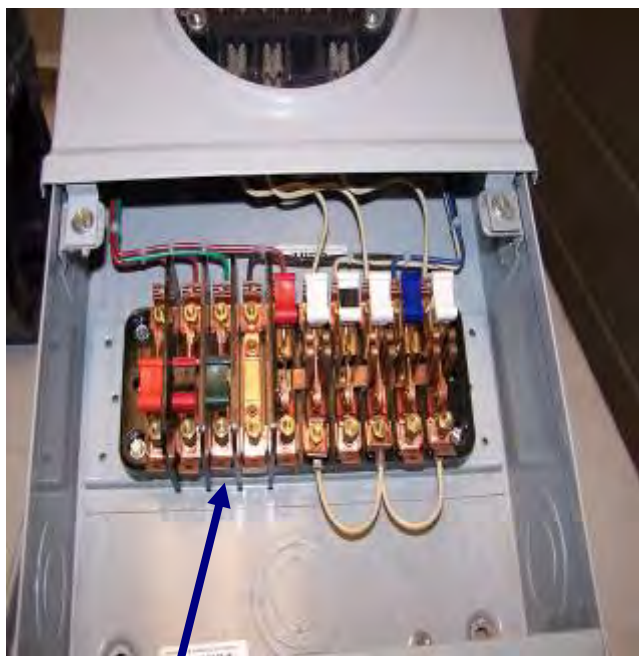
Knife blade switches can be operated to provide a shorting/bridging connection of the CT secondary metering circuit to allow for installation, replacement or removal of the meter on and energized service installation.
