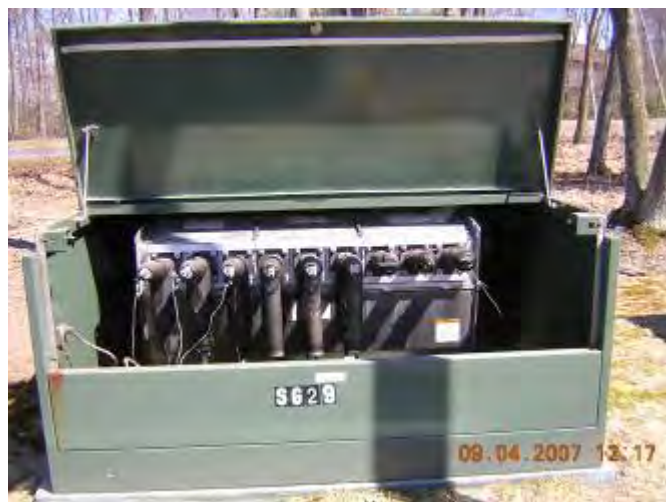
PADMOUNTED VISTA SWITCHGER
